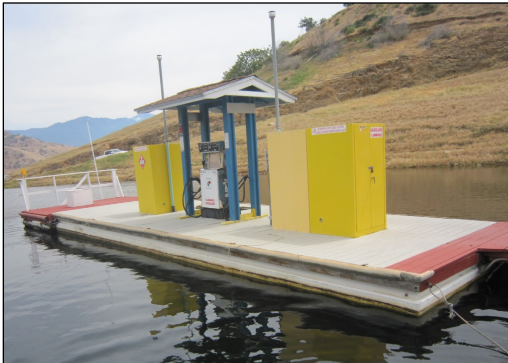
FIGURE 1-1 Floating Gasoline Dispensing Facility
