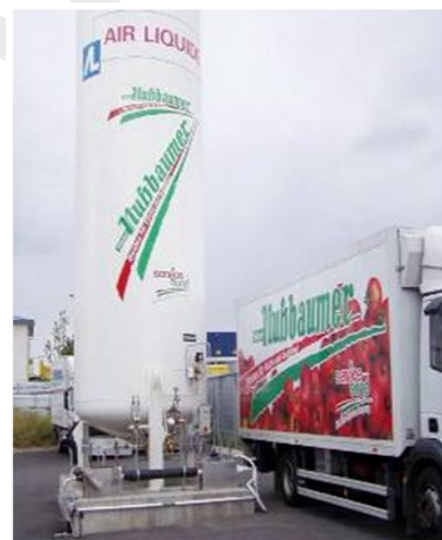
Figure III.E-14: LN 2 Fill Station (Air Liquide, 2009)
