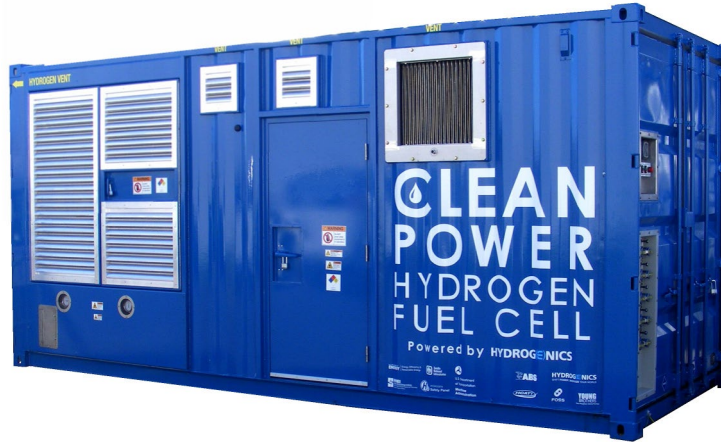
Figure III.C-5: Containerized H2 FC Generator (Hydrogenics Corp.)
