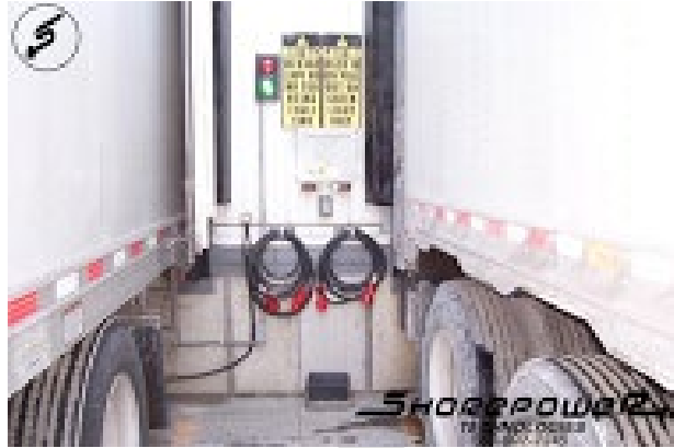
Figure III.A-3: Loading Dock Power Plugs
